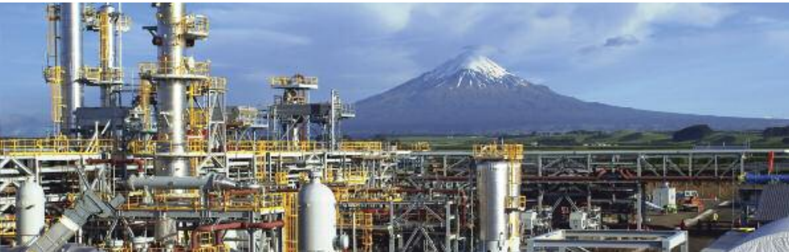
Origin Energy's Kupe project in South Taranaki on New Zealand's North Island is scheduled to come online by the end of 2009
