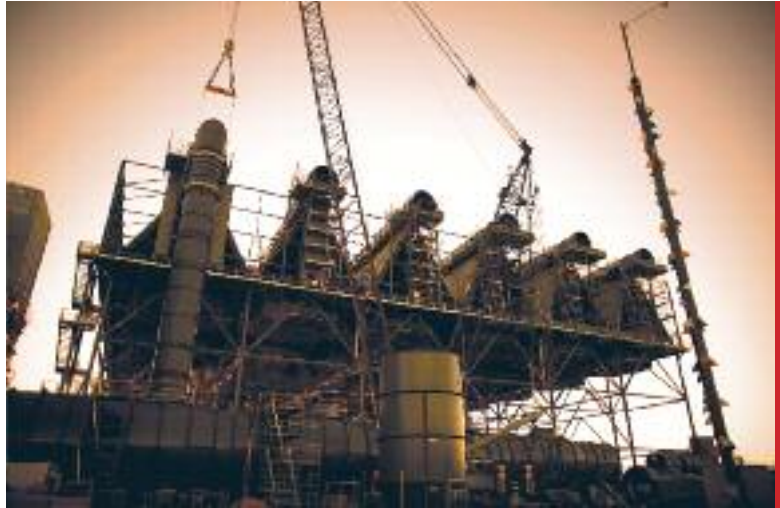
Construction of Origin Energy's 630-MW Darling Downs gas-fired power station commenced in 2007
