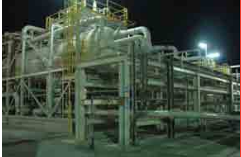
DNO's central processing facilities in Tawke.
