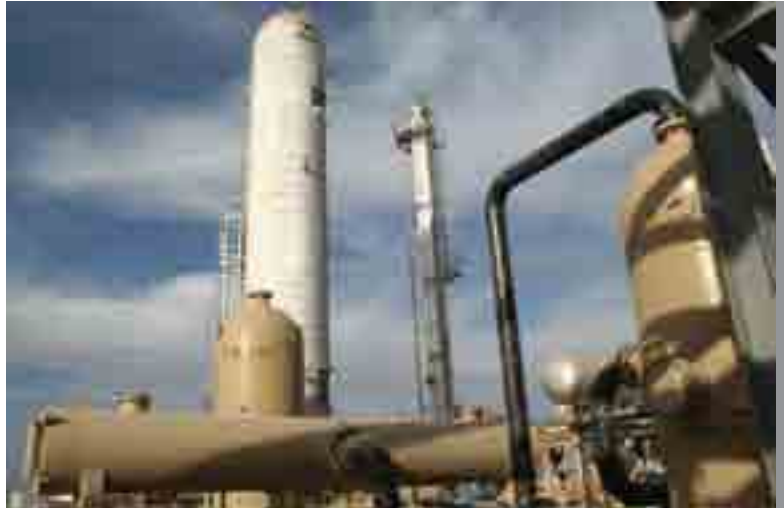
Khor Mor has been fully redeveloped, including LPG facilities, allowing the Kurdistan Region to nurture power generation capabilities for local needs and position itself as an upcoming gas export province
